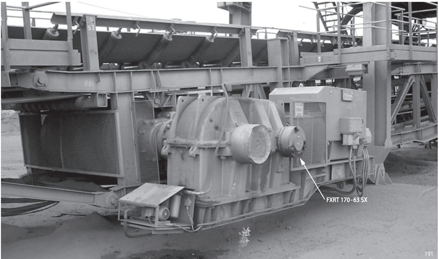
Iron ore conveyor plant in South Africa driven by three gear reducers with RINGSPANN backstops FXRT 170 SX.
